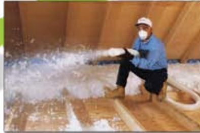
2. R42 Attic Insulation
